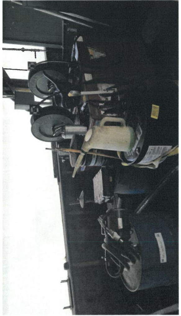
Virgin Oil - Secondary Containment
