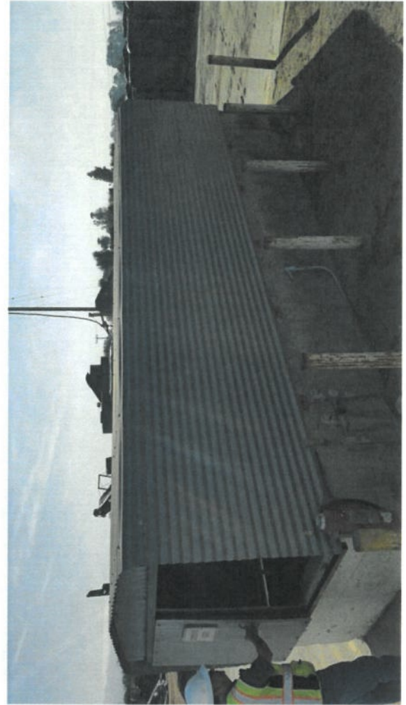
2,000 gallon Diesel AST w/ secondary containment and housing
