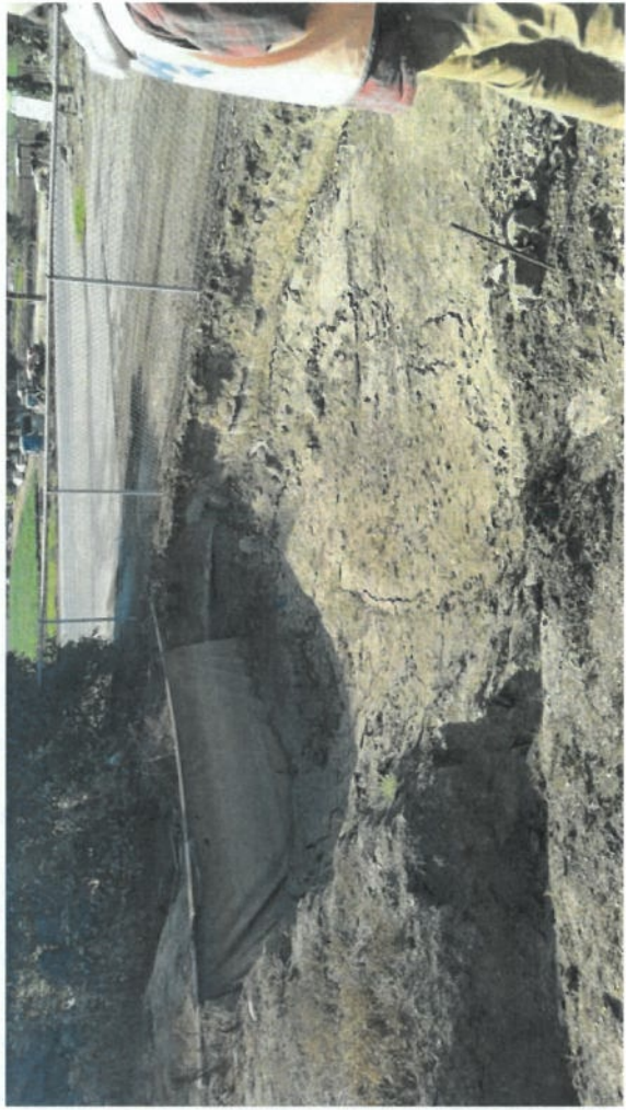
Storm water collection area
