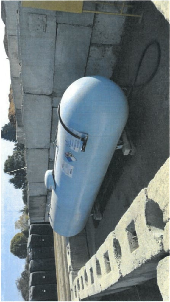
Cement Barrier Protected Propane Tank outside building 3
