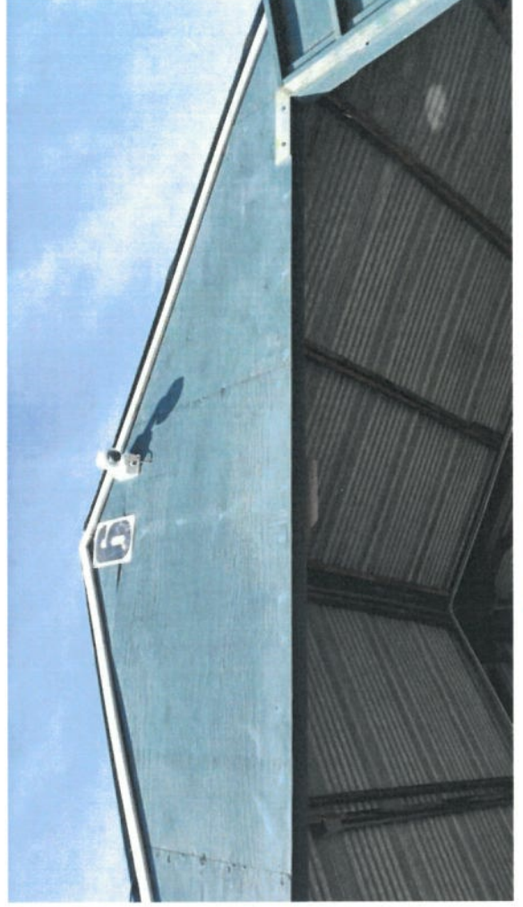
Building 6 - Metal Shop - Equipment
