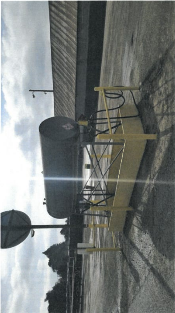
1,000 gallon Diesel AST w/ Secondary Containment
